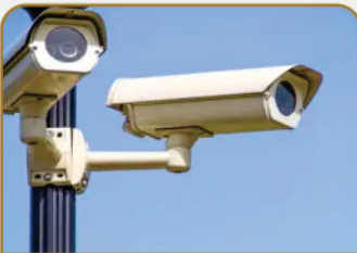
24X7 SECURITY & CCTV SURVEILLANCE
